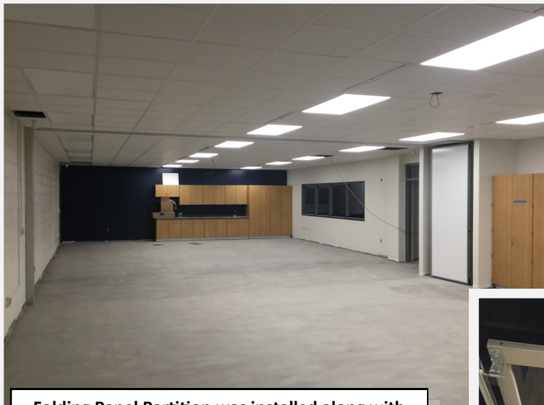
Folding Panel Partition was installed along with ceiling grid, lights, grilles, and this room has ceiling tile competed
