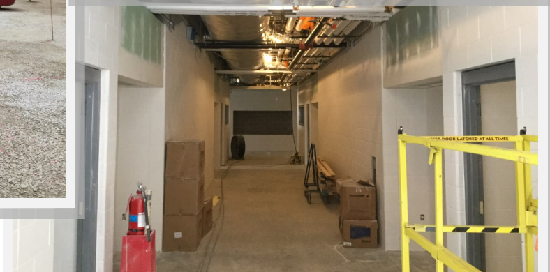
MEP Above Ceiling Rough ins are installed and insulated, taping/mudding complete, priming and painting is underway.
