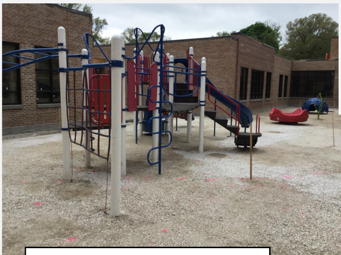
Courtyard Playground Equipment installed
