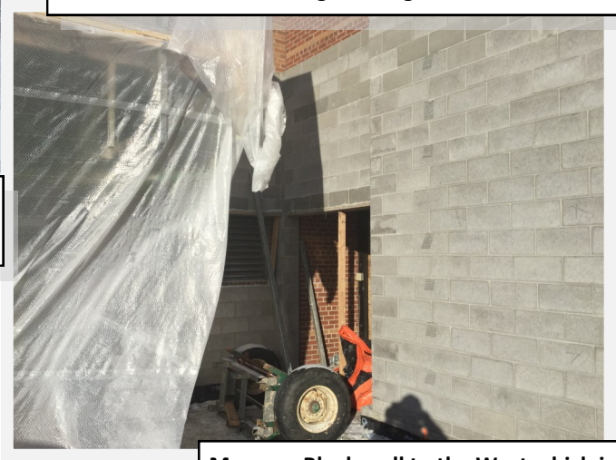
Masonry Block wall to the West which is against the existing building
