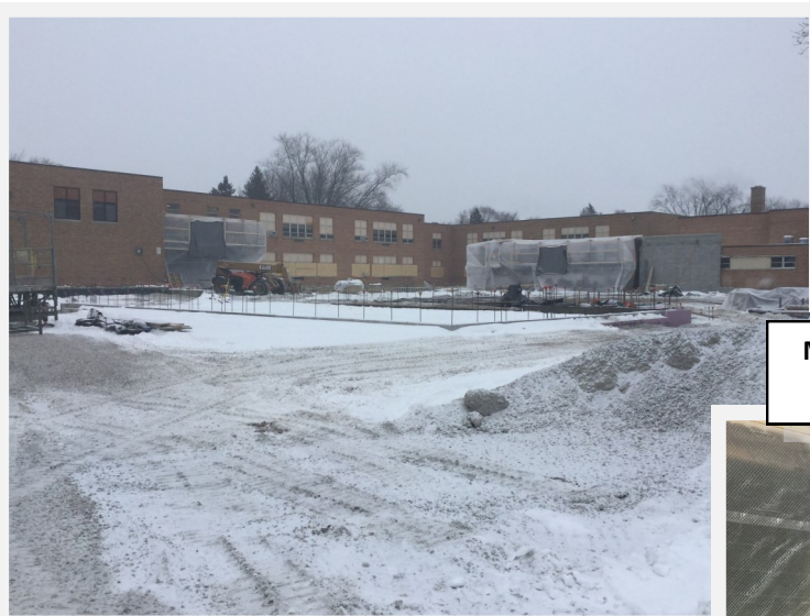
Overall Site Picture, Masonry Enclosures on either side of new addition building block walls
