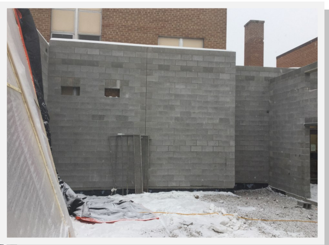
Masonry Block wall to the East which is against the existing building
