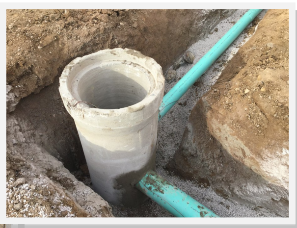
Storm Drainage System
