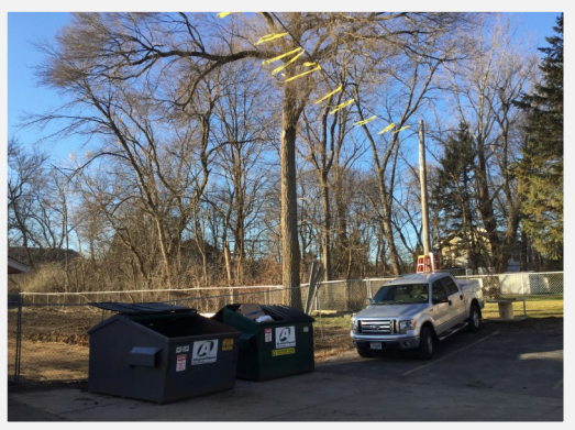
Temporary power line for construction trailers
